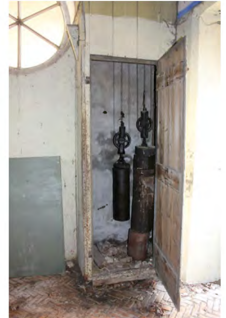
Clock weights in loose box
