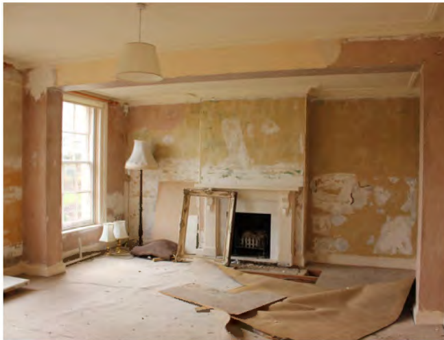
Breakfast room, formerly the butler's sitting room and bedroom. Note the raised flooring, removed wall, and relocated fireplace
