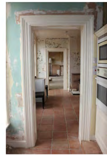
Inserted doors through GF12 to GF13. Note the foreground space was formerly a Victorian WC
